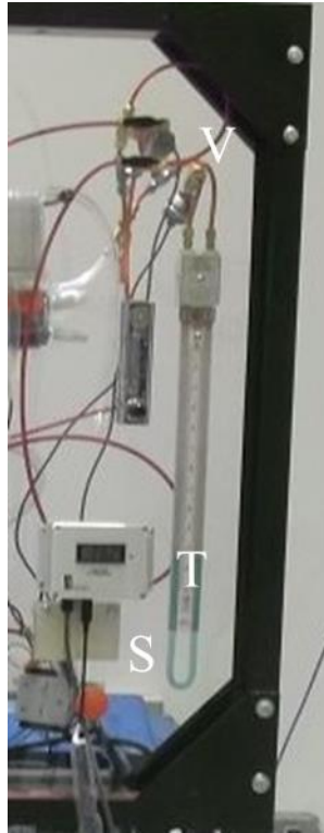
Figure 6. Oxygen-in-gas instrumentation on the control panel. Valves (V) divert the gas streams entering and exiting the membrane unit to the sensor (S). Mass percentage of oxygen in the gas stream is read on the transmitter (T).
